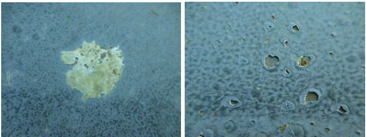
Figure 4.8 Residual oyster base (left) and paint blistering defects (right) on the vertical side.
