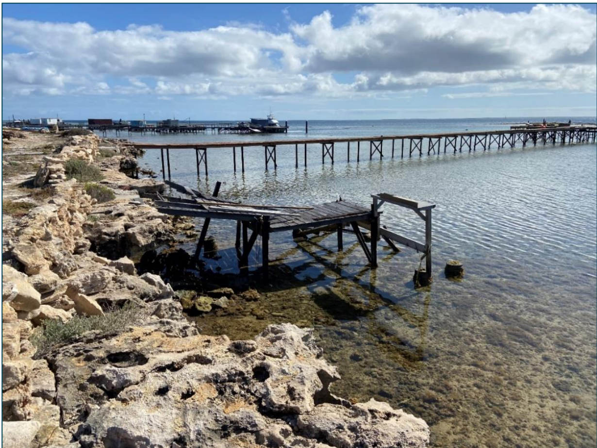
Image 39- Collapsed jetty, Rat Island, Easter Group. Credit: DPIRD, N Moore.
